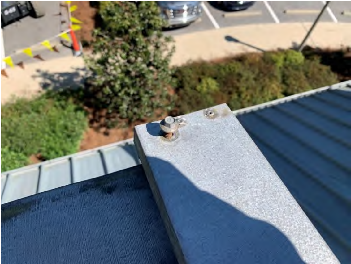
Typical rusted fasteners. Fasteners cannot be backed out due to heavy rust. They will break off. Need to seal all fastener heads and install new fasteners.
