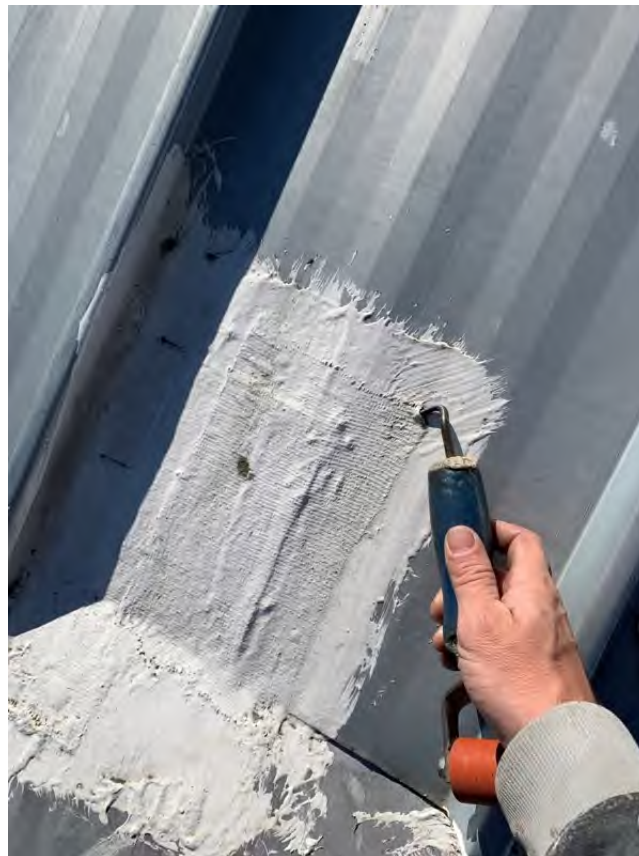
Remove old defective patches throughout G dormers and replaced with a GACO roof patch.
