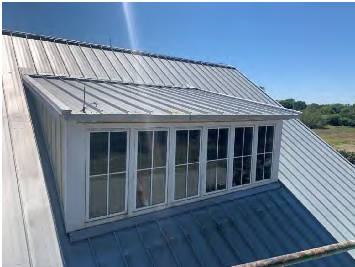
Overview of metal roofing system. Metal panels in good condition. All fasteners are rusted and in need of replacement/sealing.
