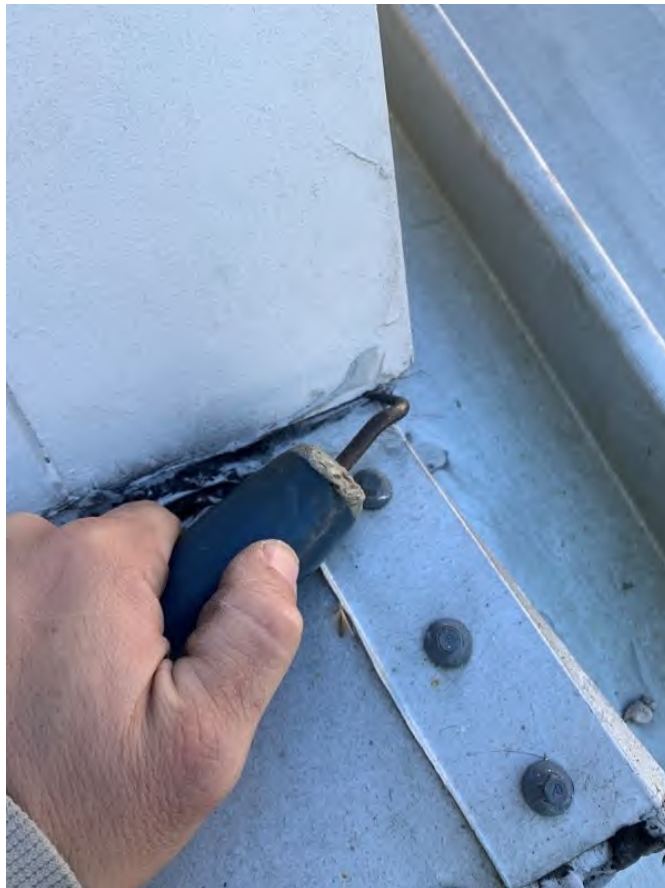
Clean and reseal all open corners and edge of dormer's.
